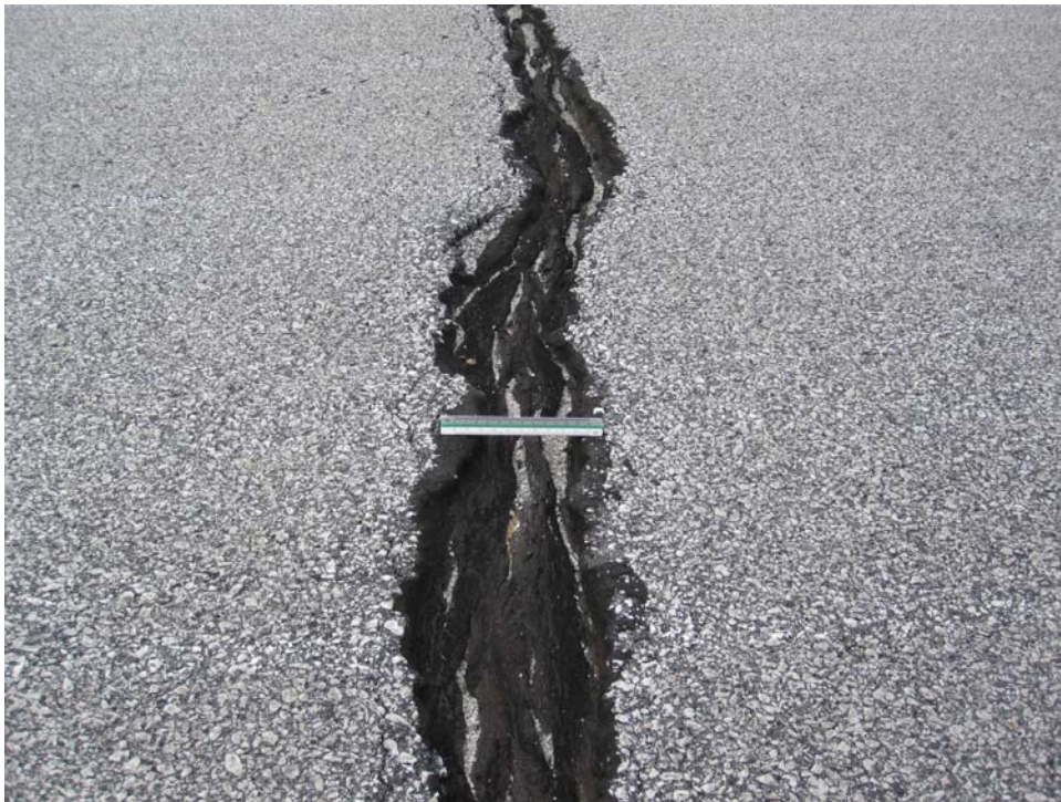
R927AB-10. High Severity Crack (Sample Unit #06).
