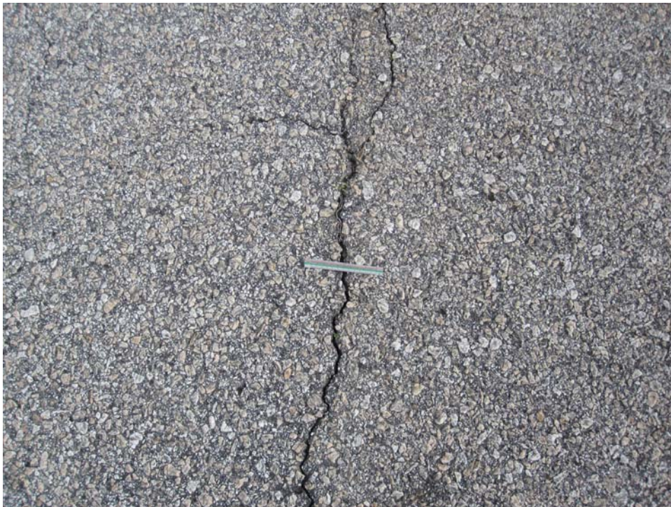
T927AB-20. Longitudinal and Transverse Cracking (Sample Unit #02).
