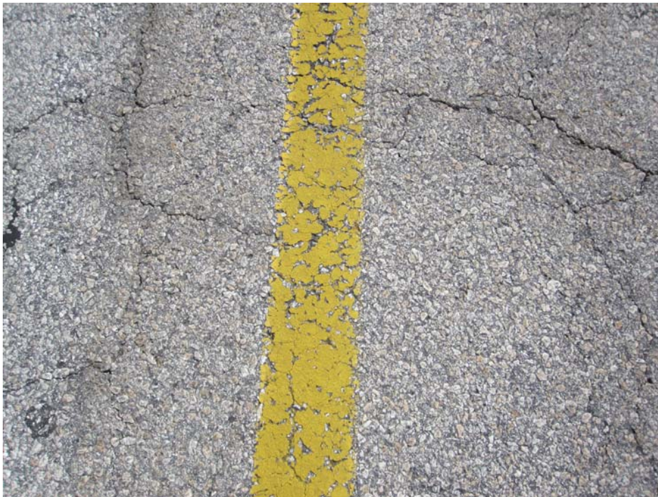
TAAB-10. Unsatisfactory Paint.
