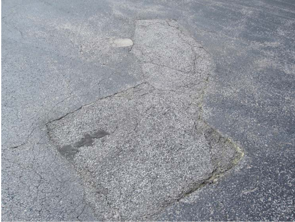
A01AB-10. Patching (Sample Unit #118).
