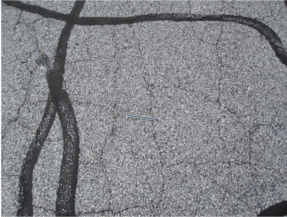
T927AB-10. Alligator Cracking (Sample Unit #02).
