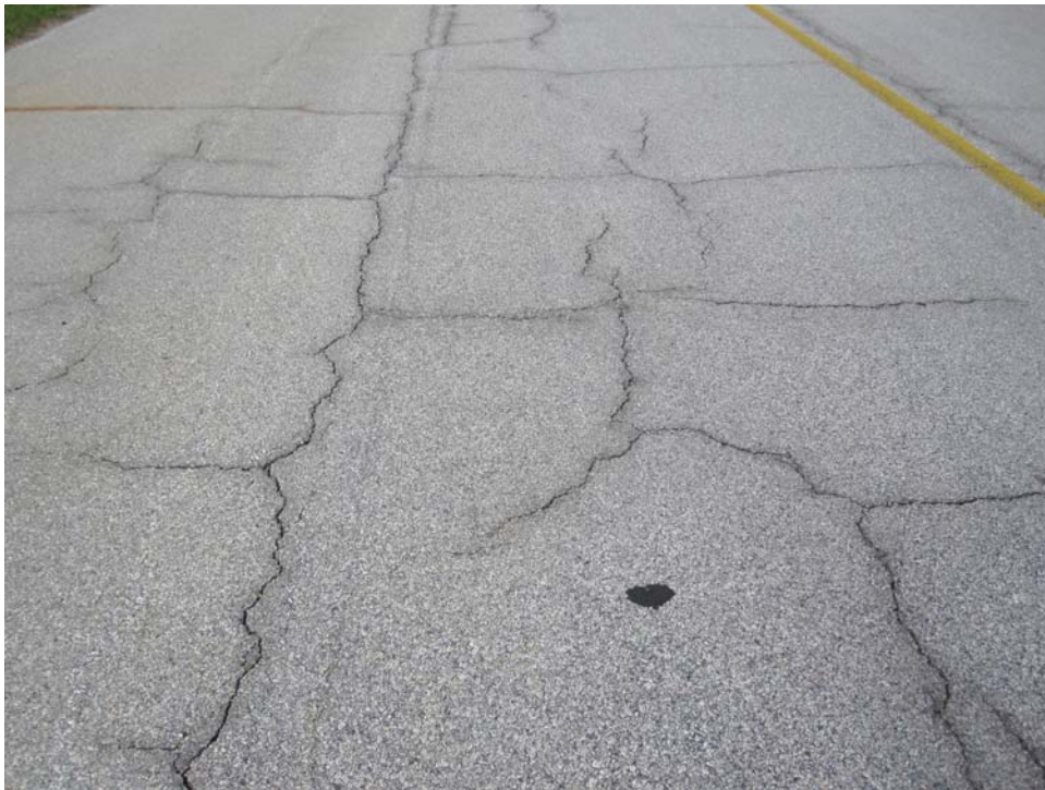
TBAB-10. Block Cracking (Sample Unit #34).
