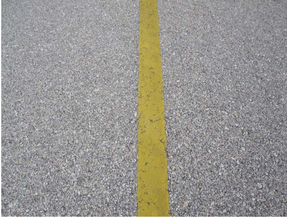
T927AB-20. Unsatisfactory Paint.
