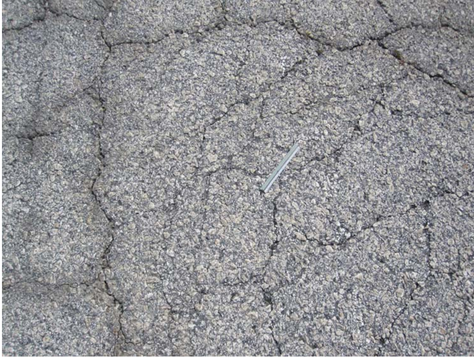
TAAB-10. Alligator Cracking (Sample Unit #07).
