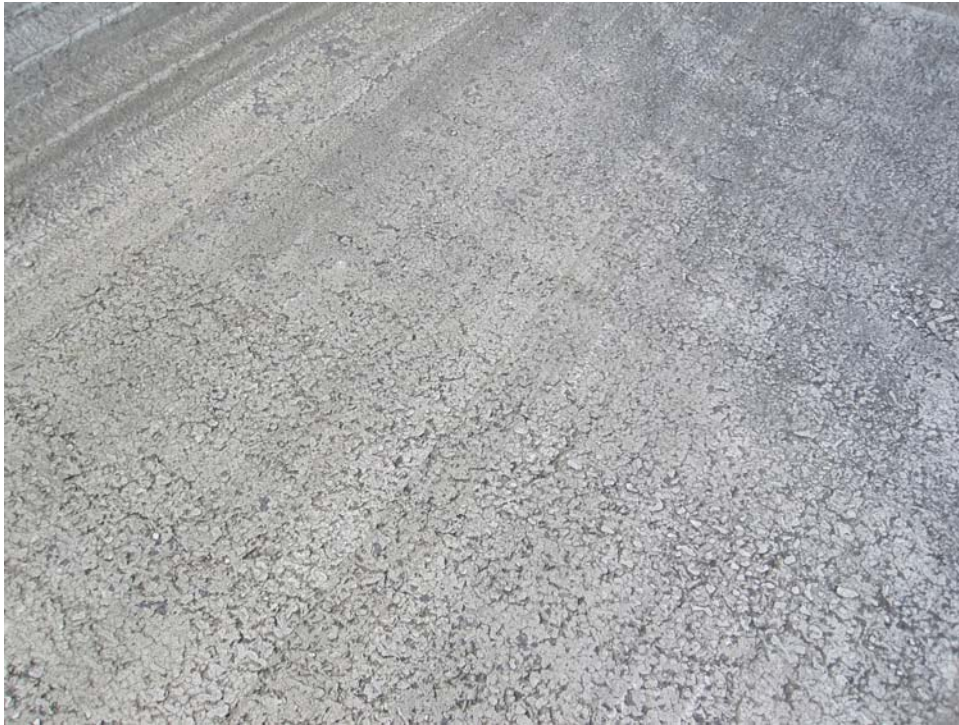
R1432AB-10. Unsatisfactory Paint (2).
