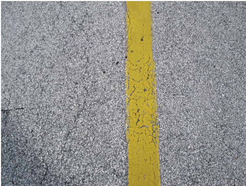
T927AB-10. Unsatisfactory Paint.
