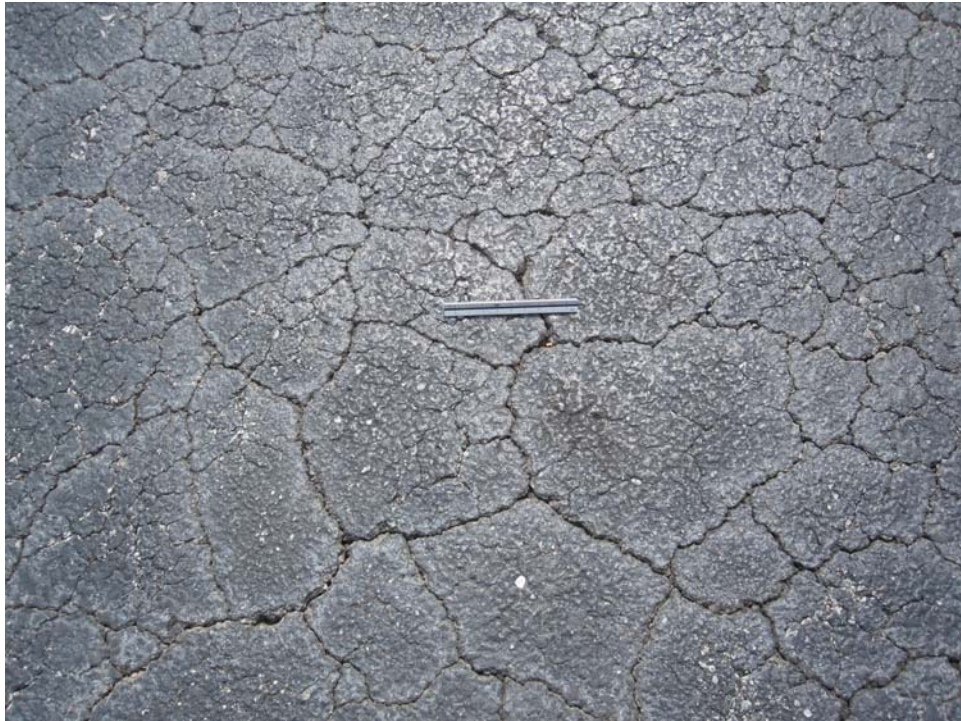
A01AB-10. Alligator Cracking (Sample Unit #58).
