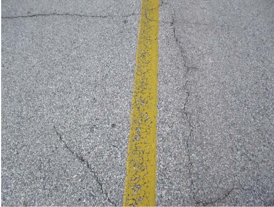
TBAB-10. Unsatisfactory Paint.
