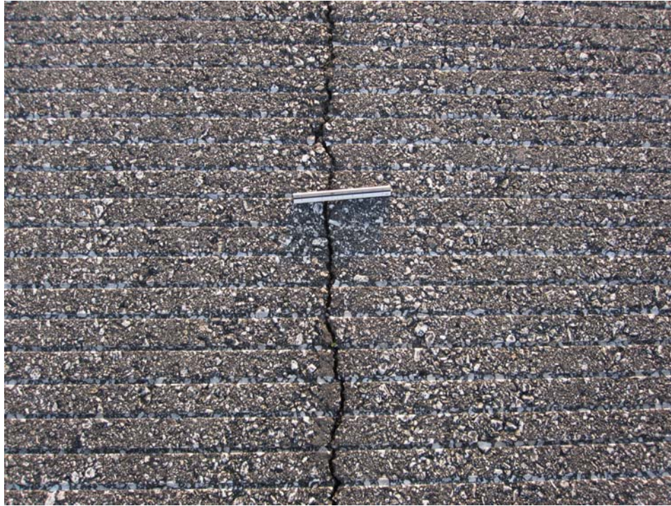
R826AB-10. Longitudinal and Transverse Cracking (Sample Unit #01).
