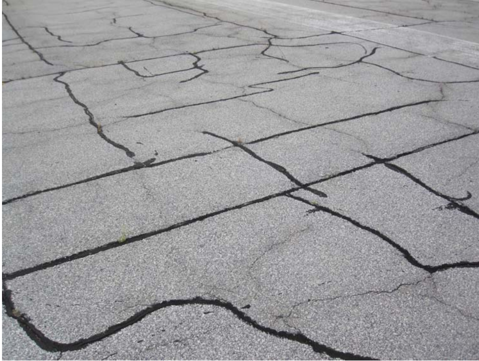
R1432AB-10. Block Cracking (Sample Unit #01).
