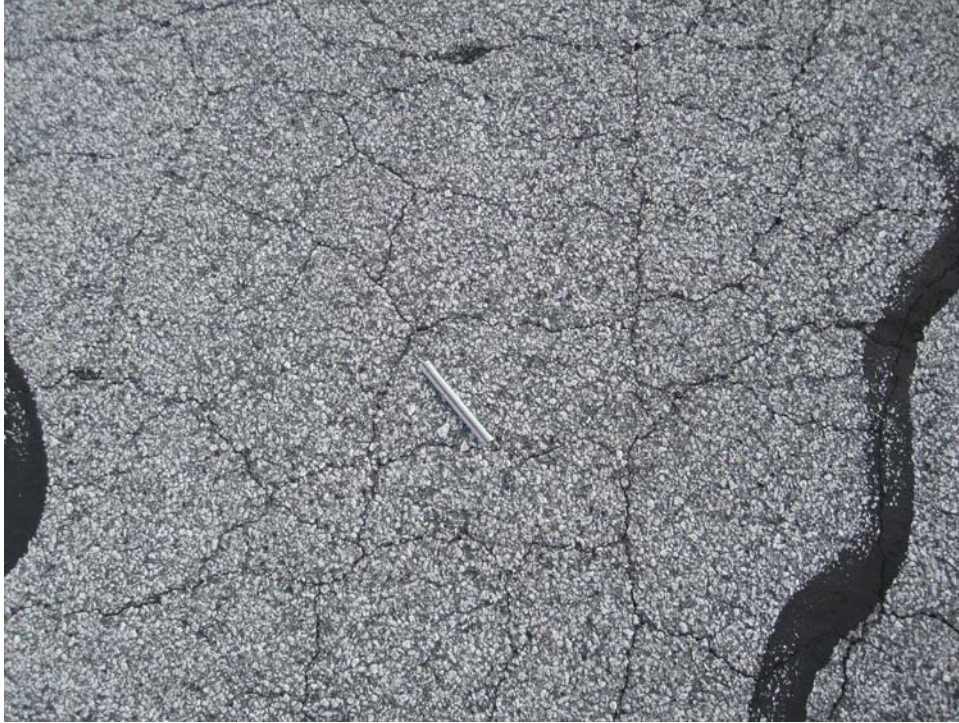
R927AB-10. Alligator Cracking (Additional Sample Unit #01).
