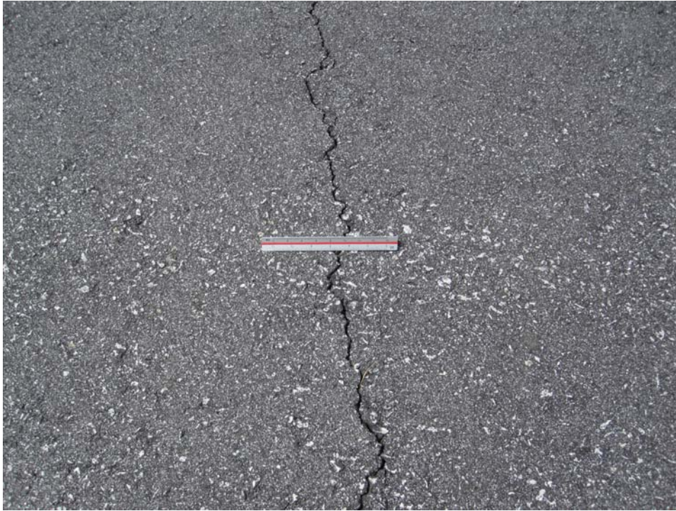
TGAB-10. Longitudinal and Transverse Cracking (Sample Unit #04).
