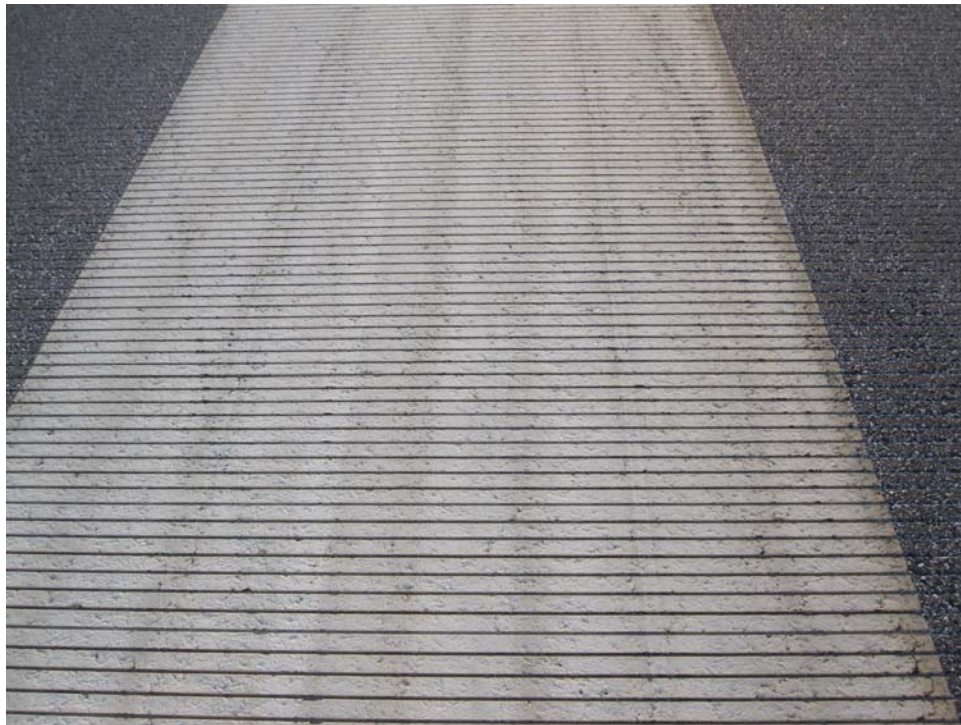
R826AB-10. Satisfactory Paint.
