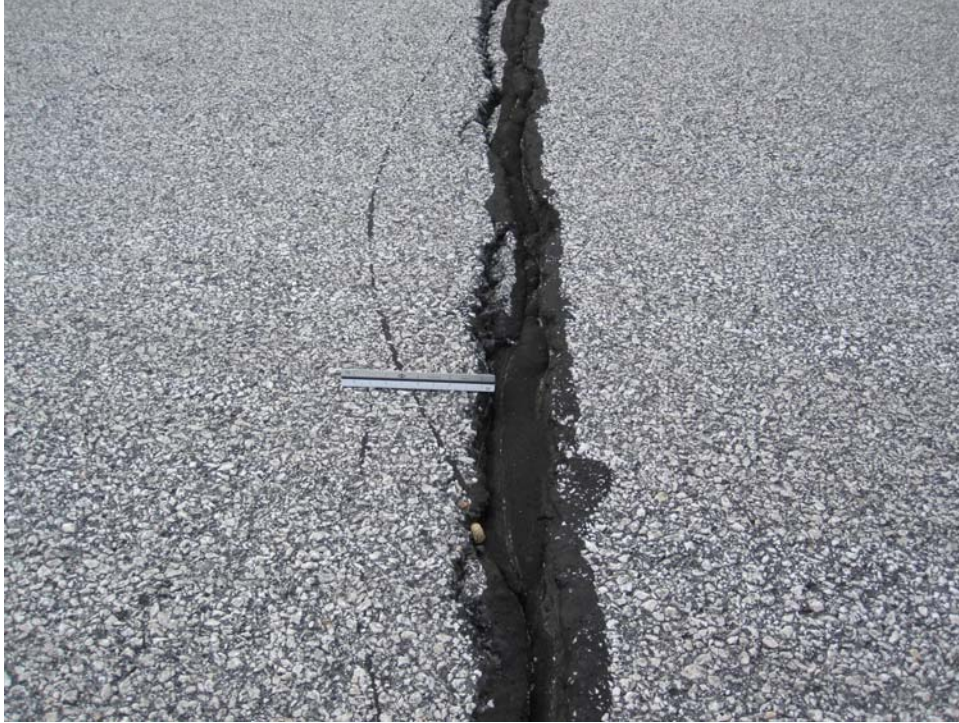
R927AB-10. Longitudinal and Transverse Cracking (Sample Unit #02).
