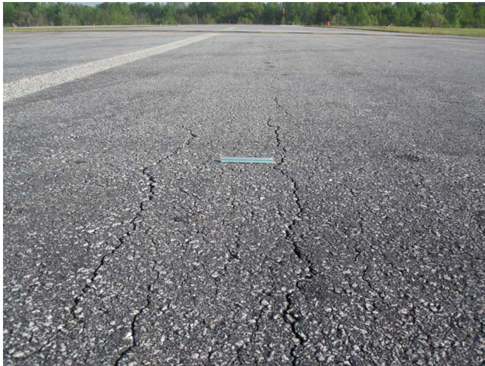
R826AB-10. Alligator Cracking and Rutting (Sample Unit #119).
