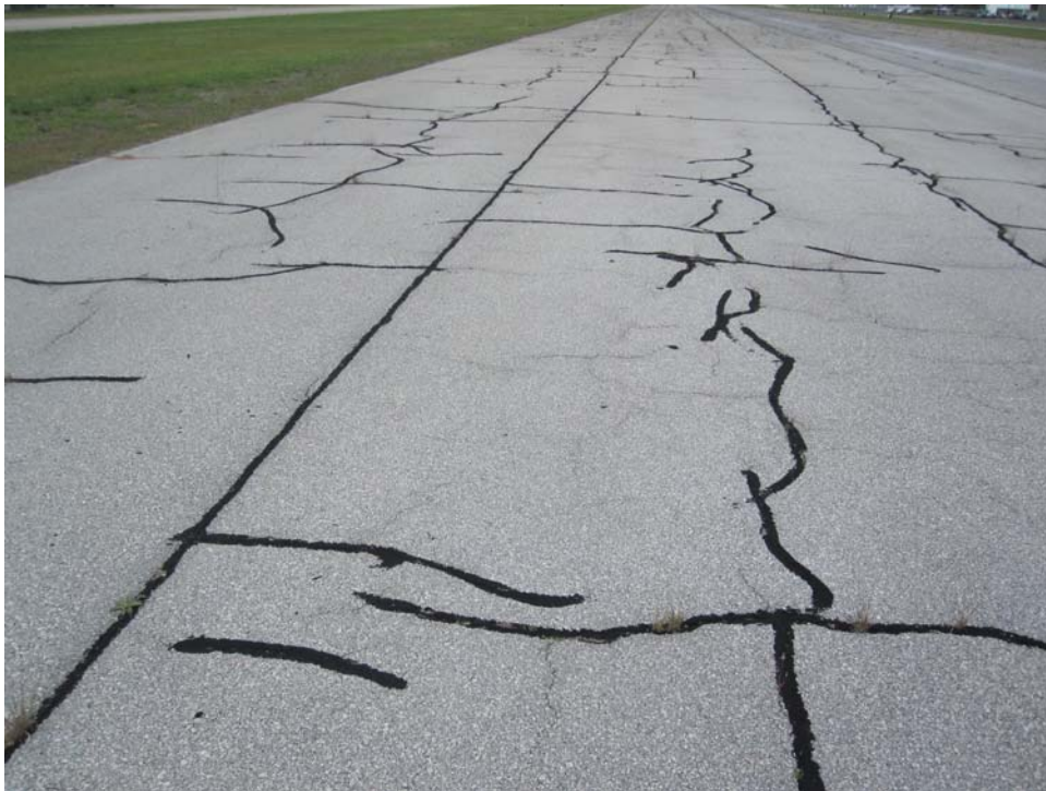
R1432AB-10. Block Cracking (Sample Unit #43).
